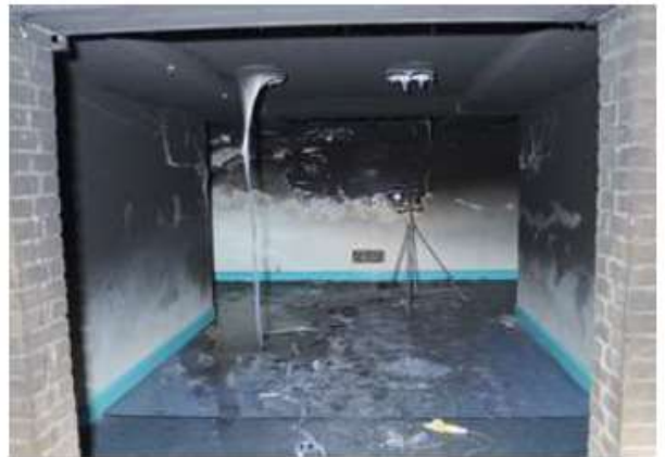
View going in through the communal entrance. Note light fittings have melted
