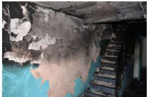
Stairwell opposite the scooter. Note; spalled plaster from the stairwell has fallen onto the stairs
